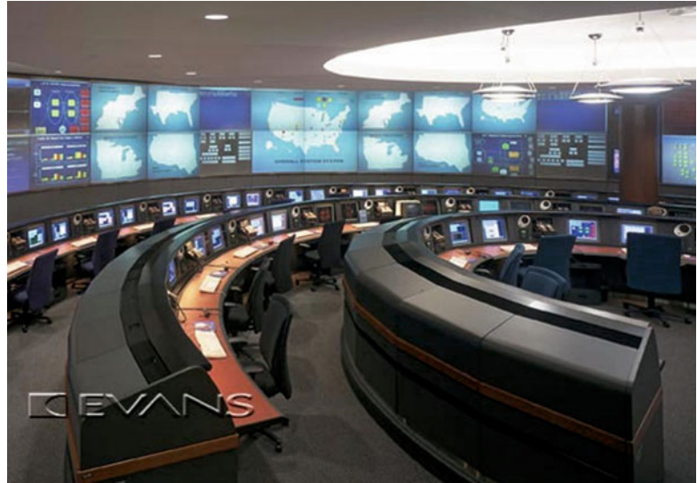
Fig. 13.3 Example of a Network Operations Center (NOC) (Reproduced with permission from Evans Consoles Corporation)
