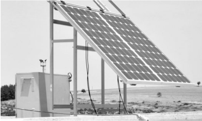
Fig. 7.13 Picture of the fixed photovoltaic panel system
